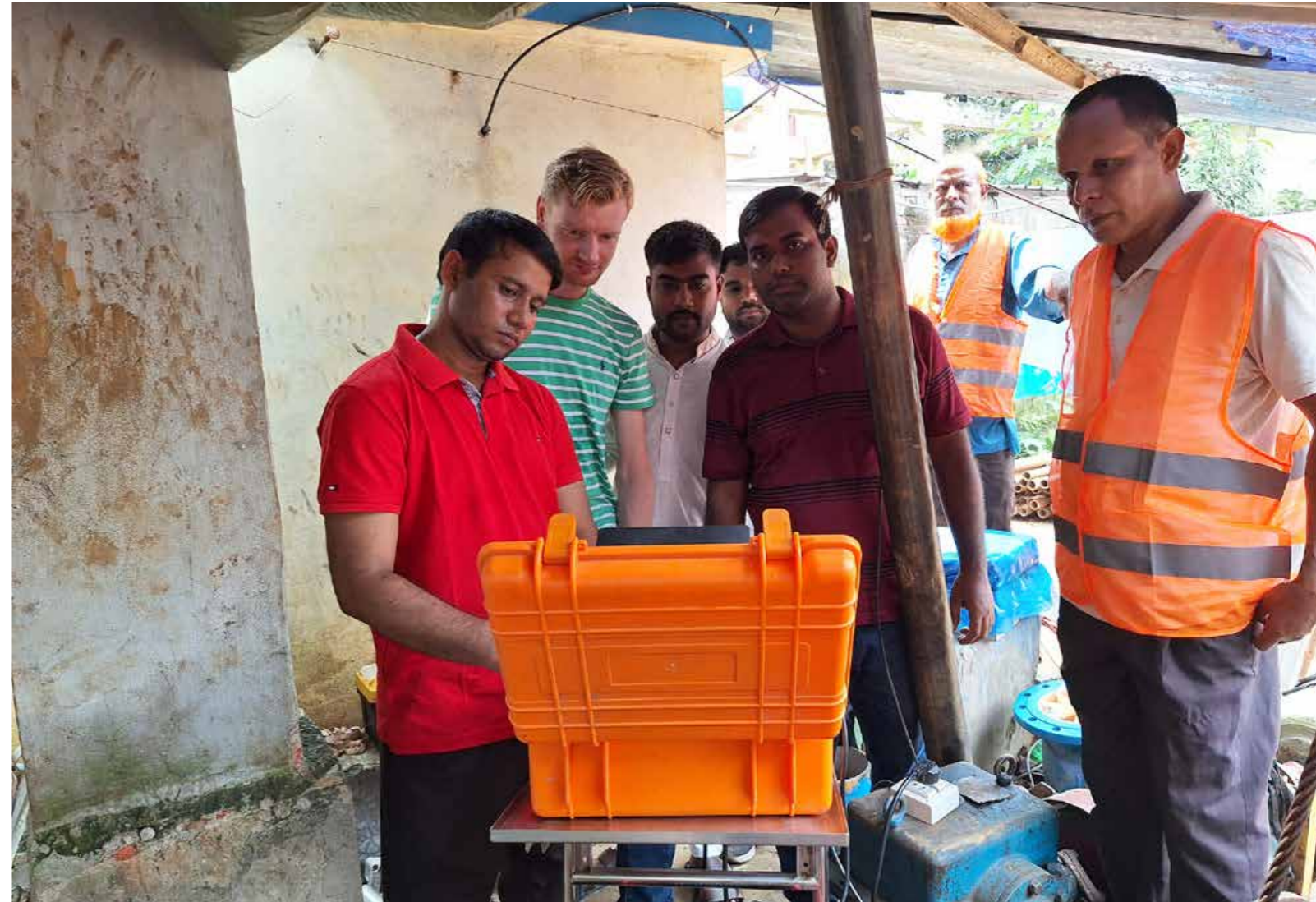
Bangladesh – Technicians perform a camera inspection to assess the condition of a damaged deep tube well in Dhaka
