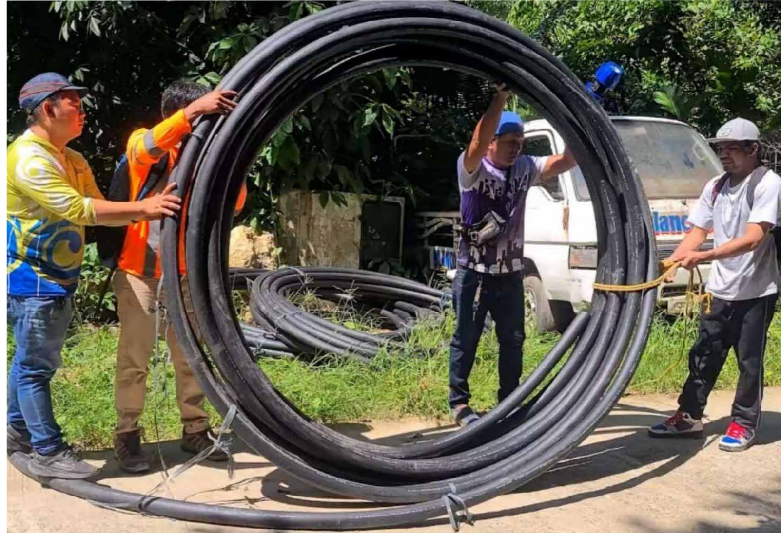
Philippines – Working on water connections in Toledo for a Water for Life project
