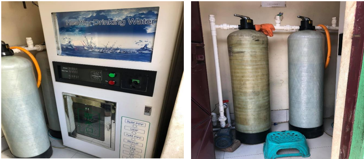
Figure 48 NC Water ATM: Robidashpara Water ATM
